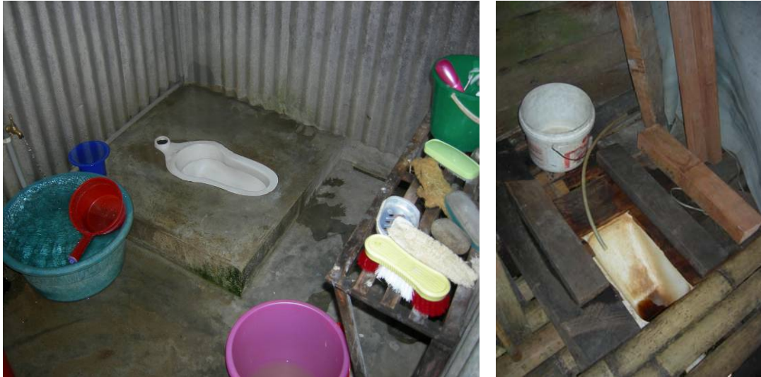
Figure 6.15 and 6.16: Squatting toilets
