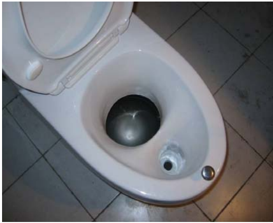
Figure 2.5: Sitting toilet with urine separation
